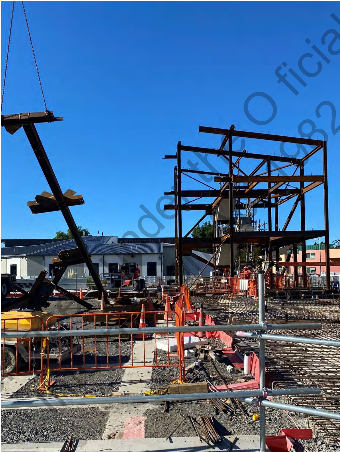
10050 – E Tū Wairua Hinegaro - Forensic Psychiatric Services Facilities Replacement, Mason Clinic, Auckland, Waitematā Structural steel frame – view from west
