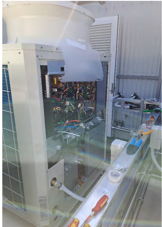
Heat pump installation
